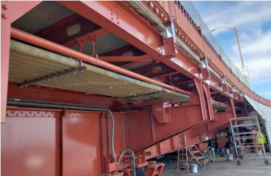
A freshly painted portion of the Golden Gate Bridge's south approach viaduct.
